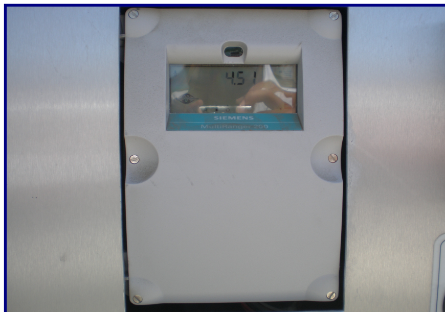
Milltronics Instrumentation on MCC Panel
