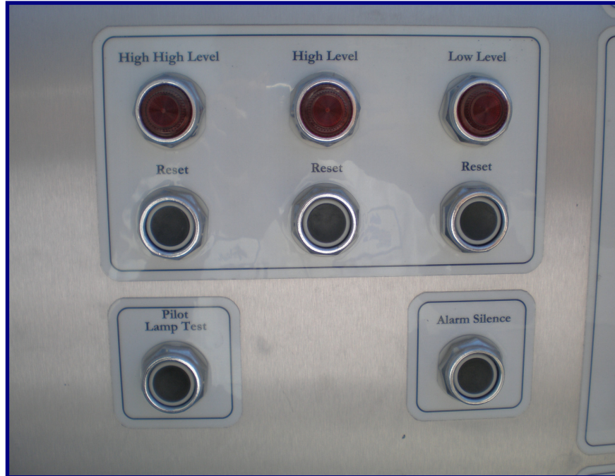
Alarm Status Lights and reset buttons on MCC Panel
