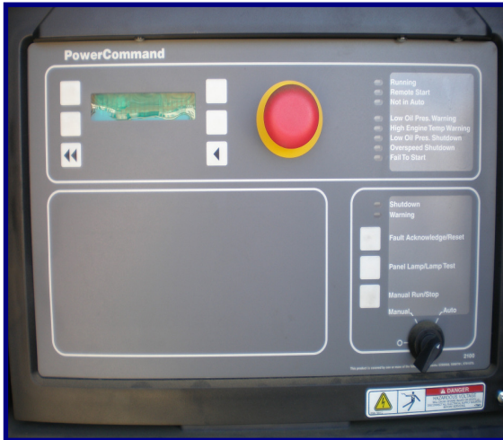
Generator Control panel
