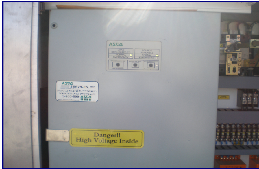
Generator transfer switch
