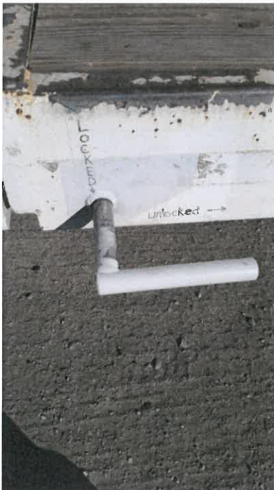
New location of the latch operator that allows for operation
