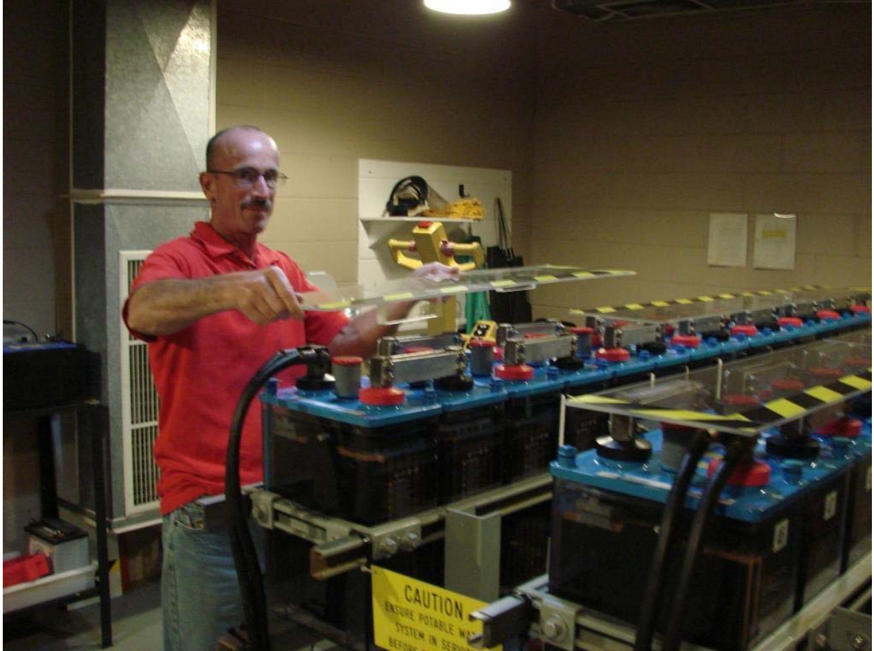
Placement of Safety Covers on Station Service Batteries
