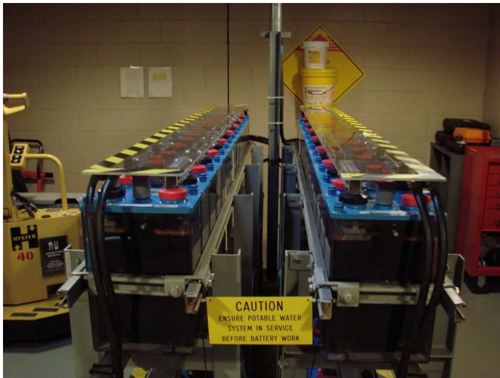
Plastic Safety Covers on Station Service Batteries
