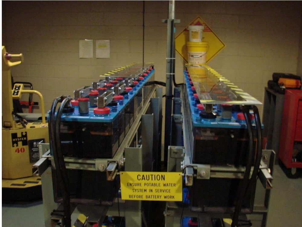
Station Service Batteries Cover and no Cover
