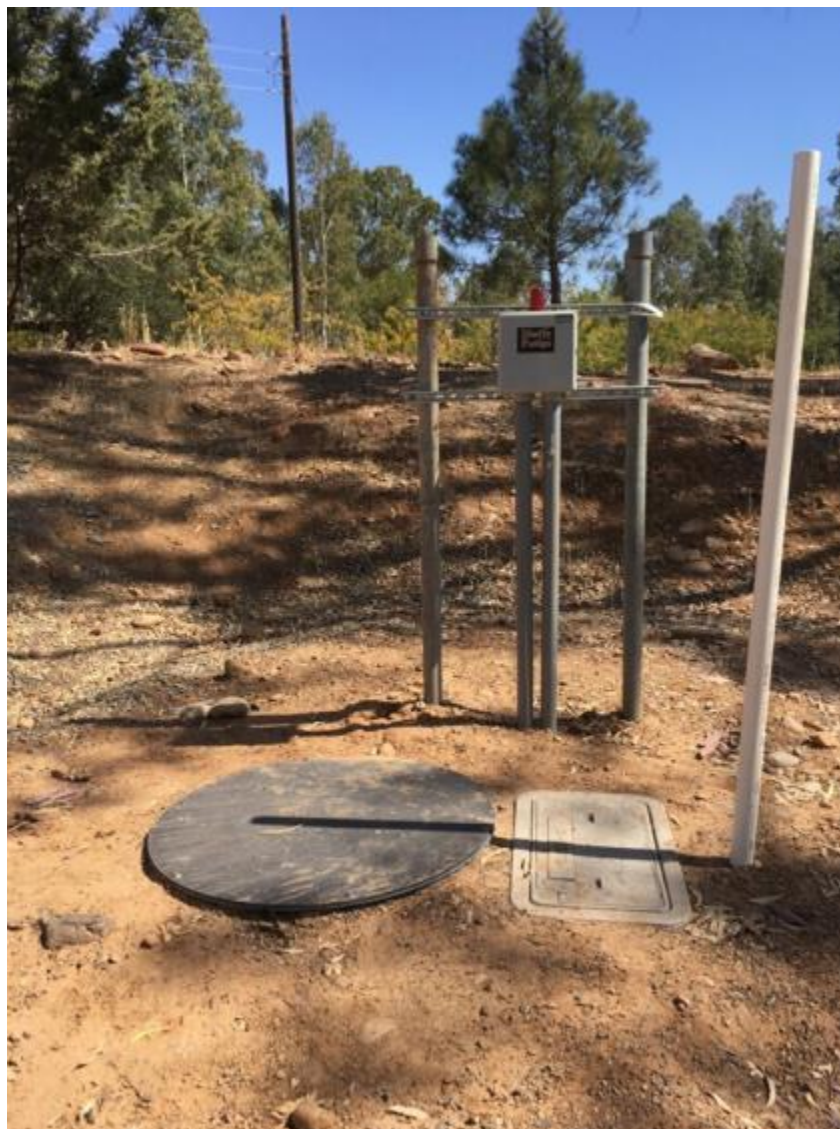
New Lift Station
