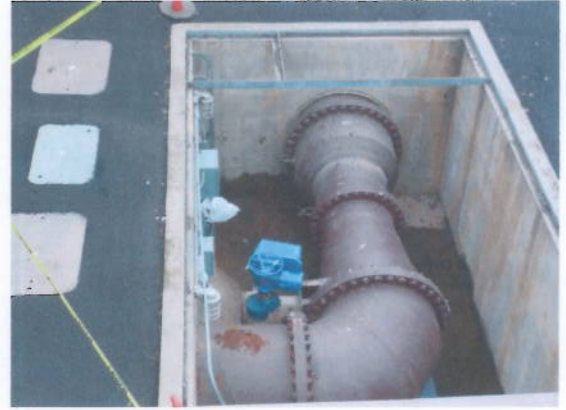
Vault uncovered showing valve controls and meter
