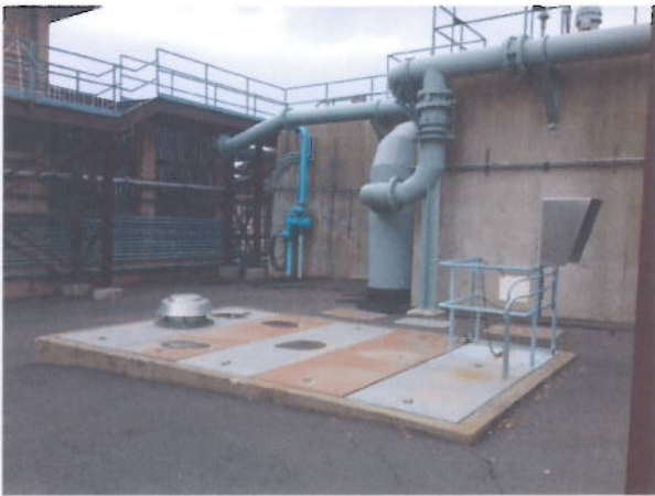
Covered vault with remote installation and meter reading on hand rail.
