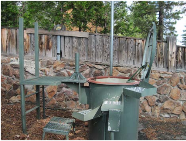
Water's Edge Sewer Station – Before
