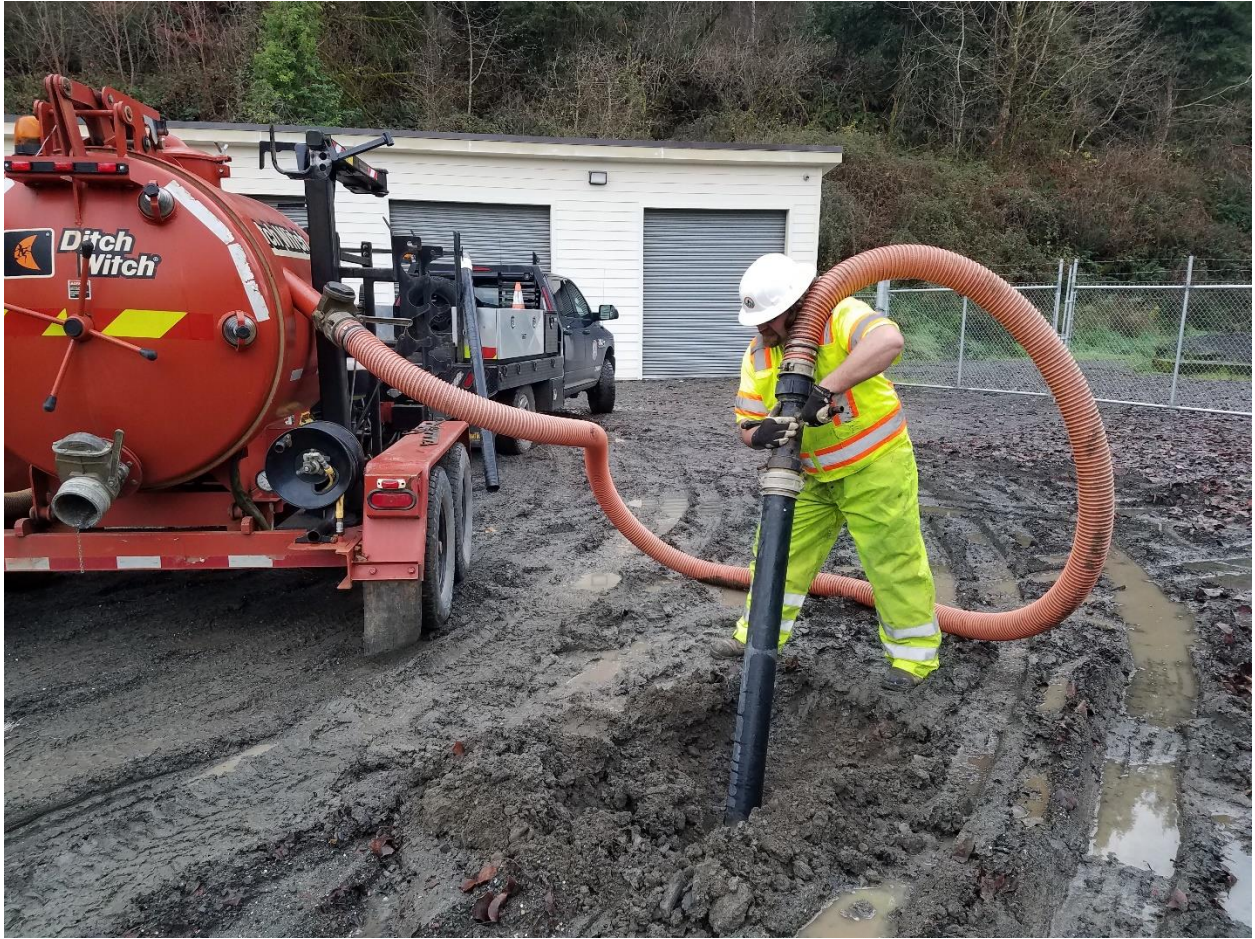
Boom not deployed, notice all the weight of the suction line is on the operator's shoulders.
