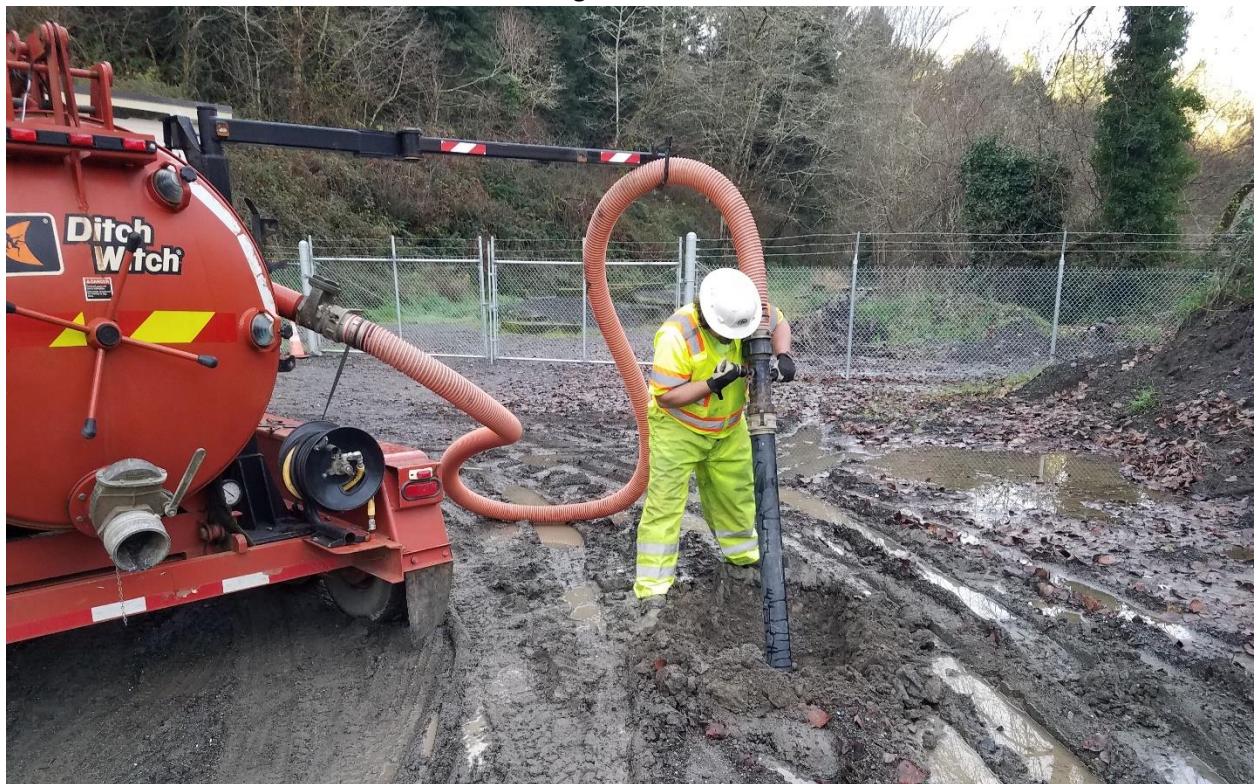
Boom deployed during operation, notice how it supports the vacuum line above the operator.
