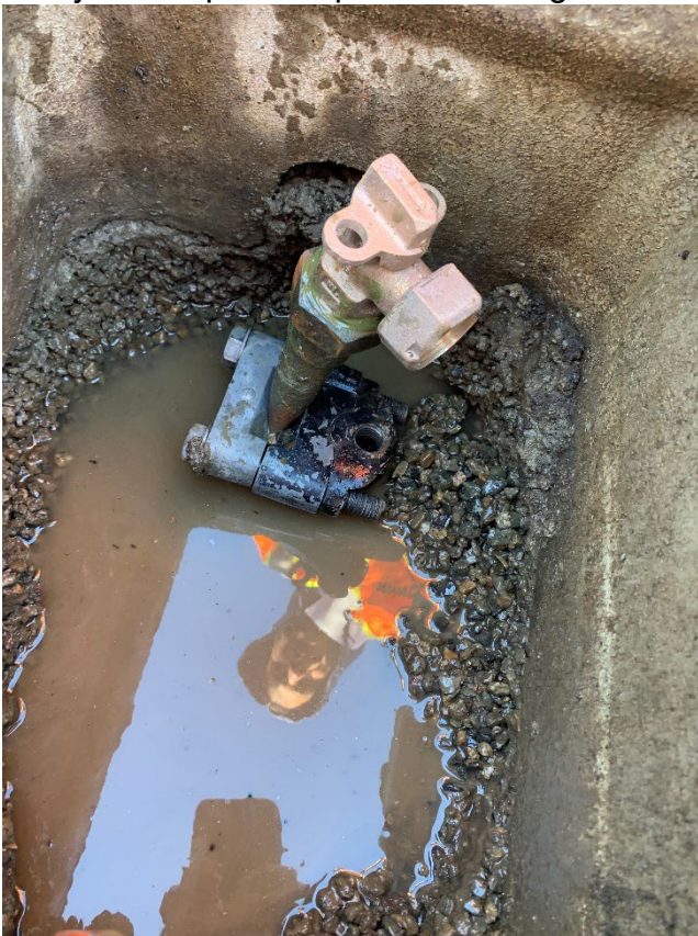
This picture shows the mini crimp in action ready to crimp and replace a leaking valve. Water is on at this point.
