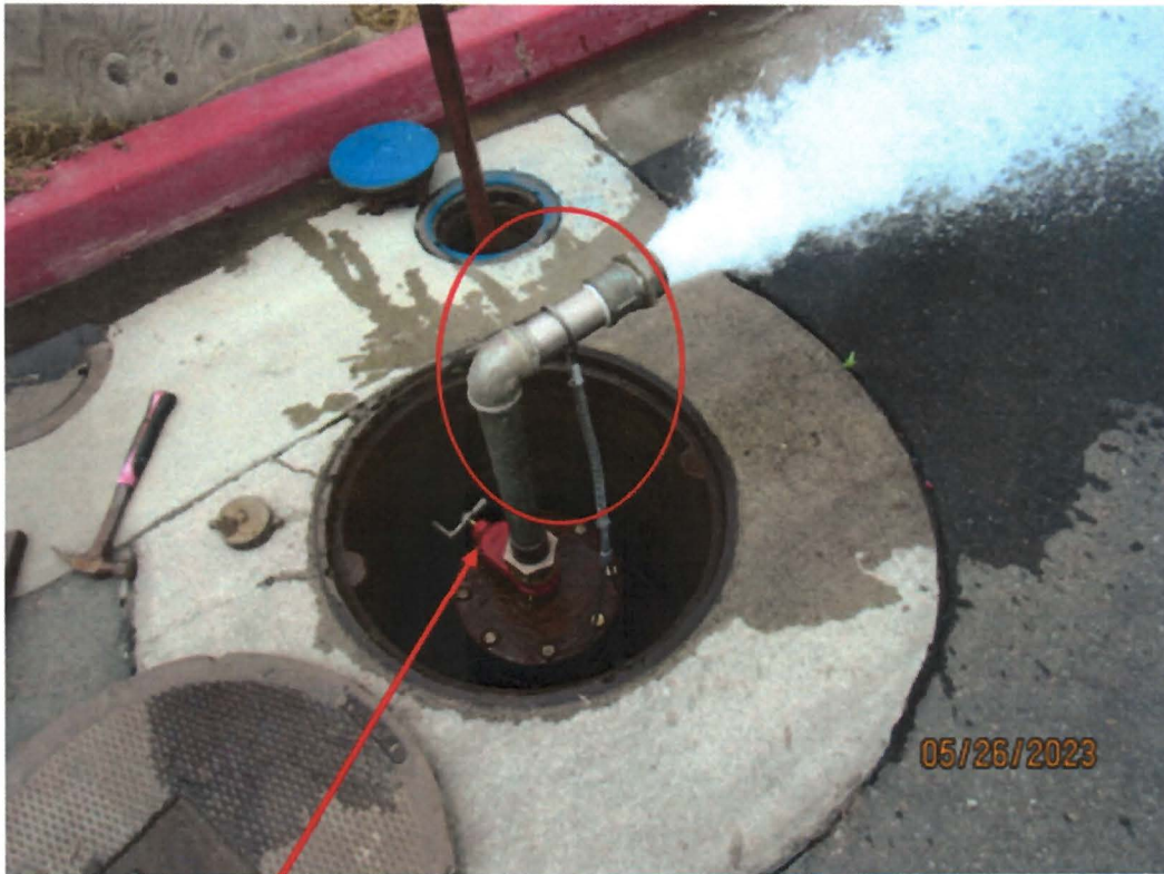
photo of the new restraining system in operation
