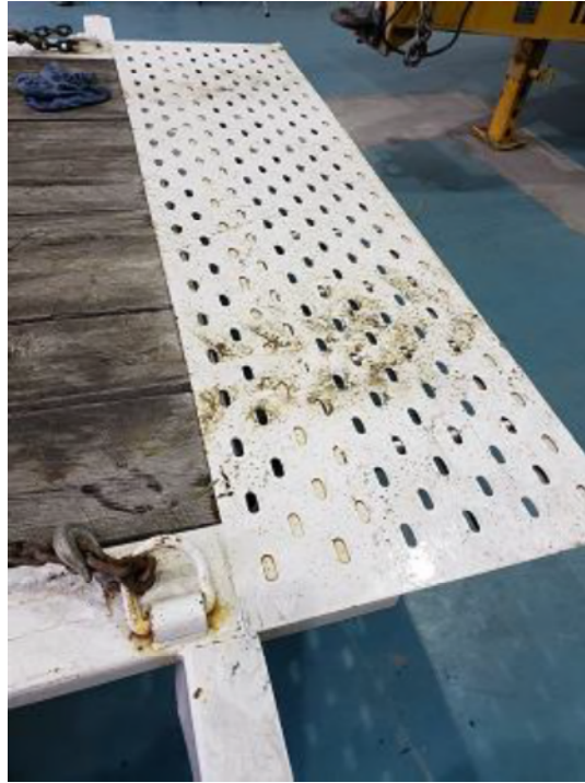
Before Coating Painted Surface – Slippery When Wet.
